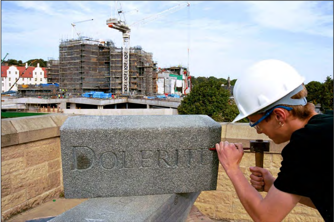
A section of kerbing, the first 'named' stone at the Scottish Parliament (under construction in the background), which will be set in place sometime in 2004. BGS image. IPR/46-32C British Geological Survey. © NERC. All rights reserved.
