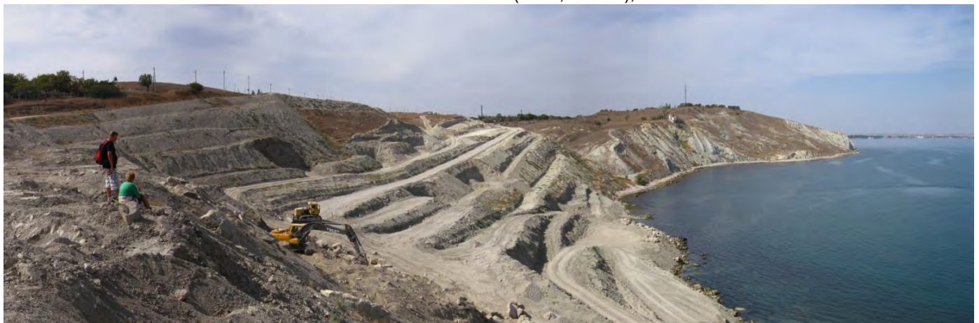
Fig. 2. The scale of excavation works is shown on sea conservation zone (photo Yu. Veklich)
