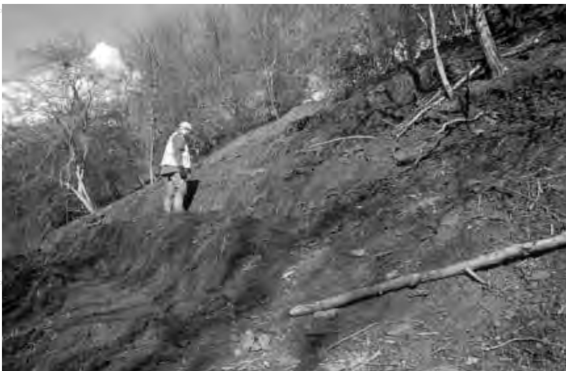
Tilton Railway Cutting showing terracing of outcrop created during vegetation clearance (Photo Mick Murphy)
